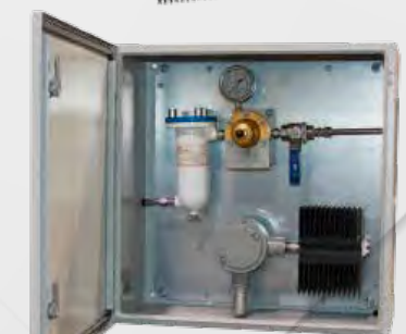
XPAS Panel Heater Mounted In a Control Panel
